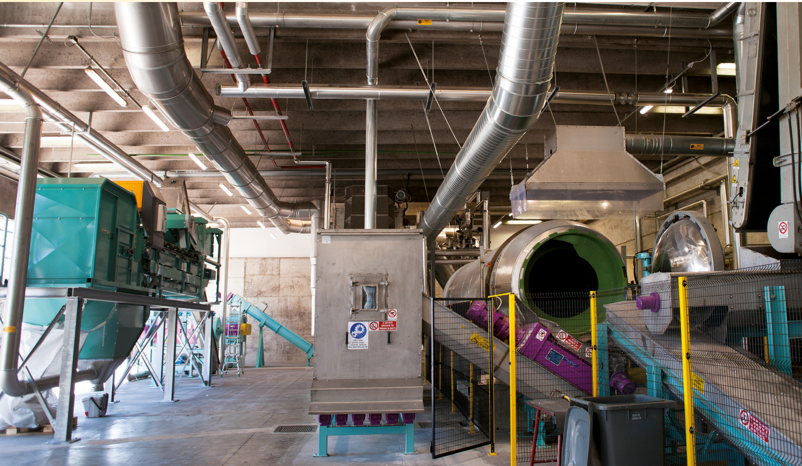
Figure 2 – Overview of the AHP waste recycling plant
